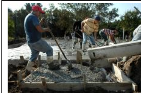
Photo by Sam Wolfe Gustavo Olivo, left, and members of the crew from Jones Masonry of Vero Beach on Wednesday level out the foundation for a home that will be built for Martha Rainey on State Street in Fellsmere. On Saturday, crews will be building two homes in one day — one for Rainey's family and one for Pamela Jefferson's family
